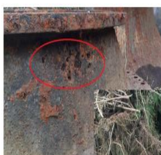
Pitting on outside surface of impeller casing
