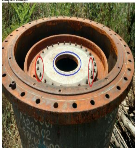
Pump Casing fasteners rubbing and cutless bearing housing along with casing material (Blue color) found complete damage.
