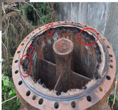
Through hole to suction casing assembly at various locations
