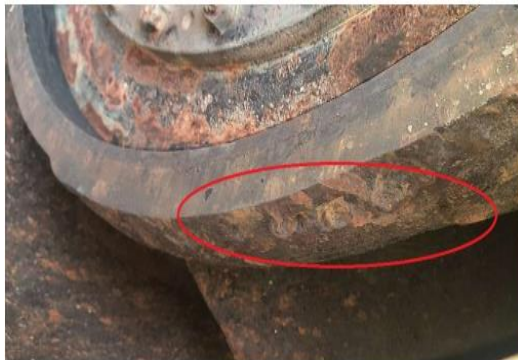
Pump casing inside surface pitting at various locations
